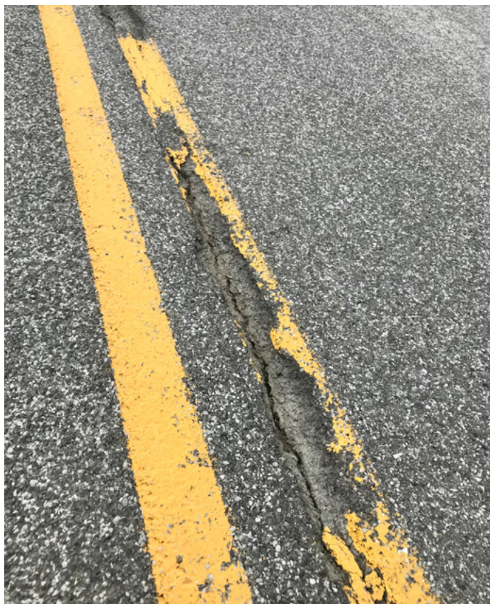
Joint deterioration before Mastic One repair
