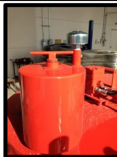
Figure 5.2 Heating Oil Overflow Tank
