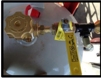
Figure 5.4 LPG Tank Valve
