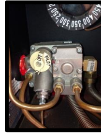
Figure 5.6 Pilot Control in Pilot Position
