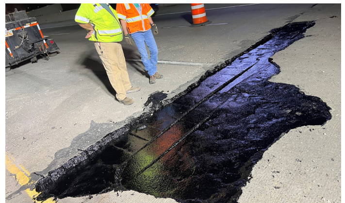
The first lift of Mastic One has been placed and is cooling before next and final lift to be installed. UDOT installed the Mastic One on all edges during the first lift to ensure a waterproof bond on all surface area of the repair.
