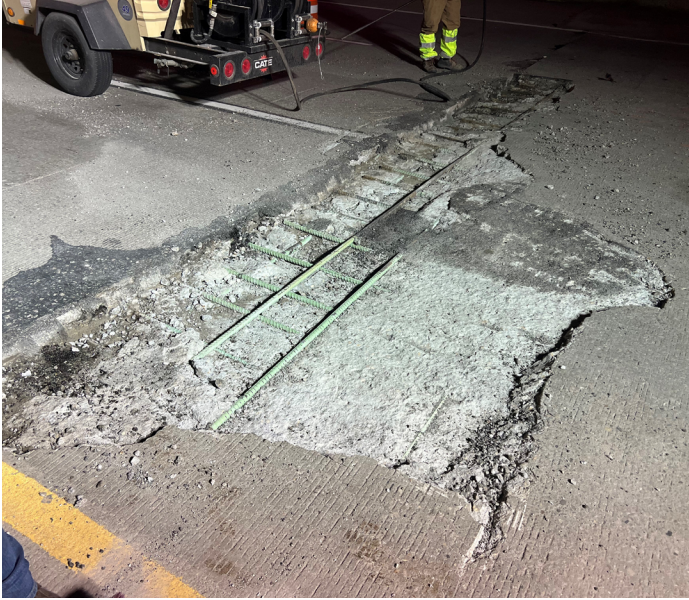
UDOT removing multiple existing patch repair materials and demolishing unsound concrete to ensure Mastic One material adheres to sound pavement.
